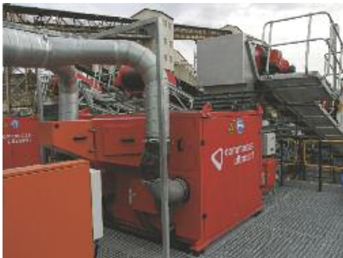
TOMRA Sorting Solutions installation at Gold Fields' Kloof gold mine: PRO Secondary COLOR
